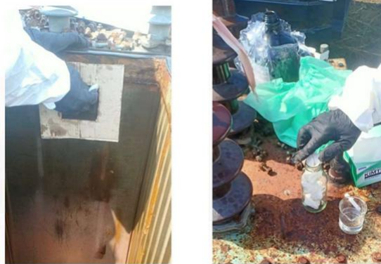
Figure 9 Transformer Offline Oil Sampling for PCBs Test, 2024
