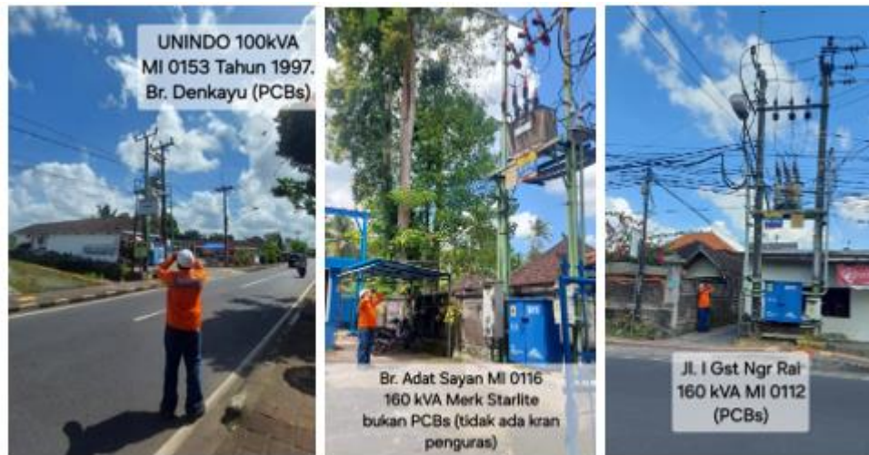
Figure 7. Transformer Online Oil Sampling for PCBs Test, 2024
