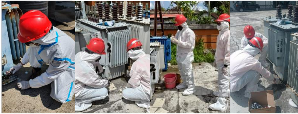
Figure 7. Transformer Offline Oil Sampling for PCBs Test
