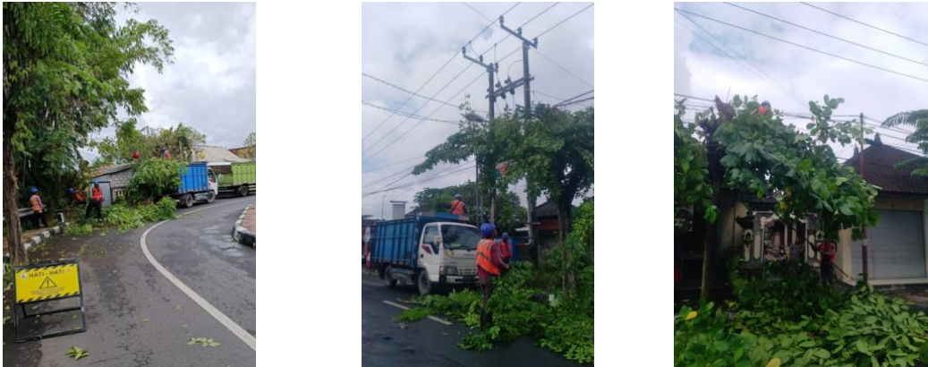
Figure 3. Tree Trimming Around Power Lines
