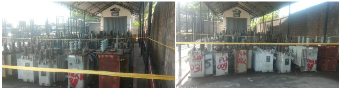
Figure 8. Transformer Containing PCBs Storage Area
